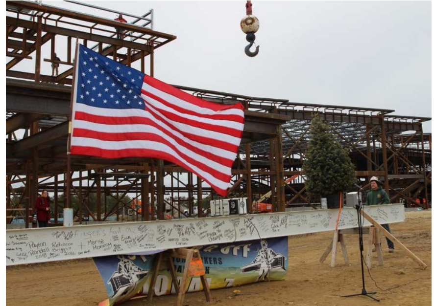
Executive Director Jack McCarthy attended the “Topping Out” Ceremony for the new Plymouth South High School project on February 23, 2016.
