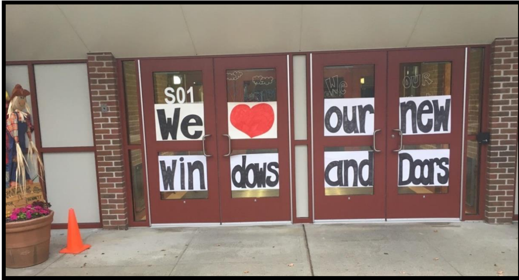
The photo above was received from the Edmund Hatch Bennett School in Taunton, a 2015 ARP Invitation. The project was completed in September 2017 and included repairs to the Roof, Windows, and Doors.
