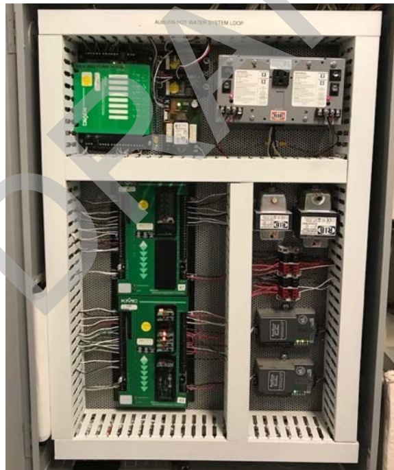
Figure 17. Retained KMC Controllers
