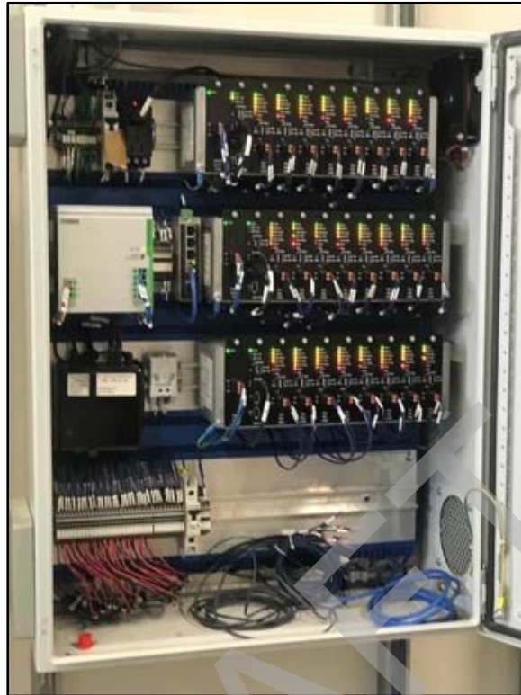
Figure 15. Eaton Lighting Control System
