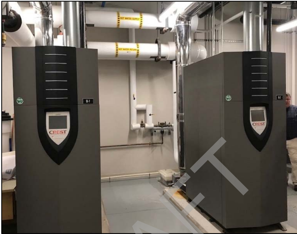
Figure 6. Two 2.5 MMBtu per Hour Lochinvar Condensing Boilers
