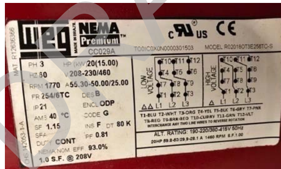
Figure 11. Motor Nameplate from Heating Hot Water Pumps
