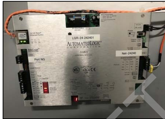
Figure 16. ALC Primary Controller
