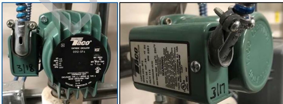
Figure 14. Service Hot Water 1/8 HP and 1/35 HP Circulator Pumps
