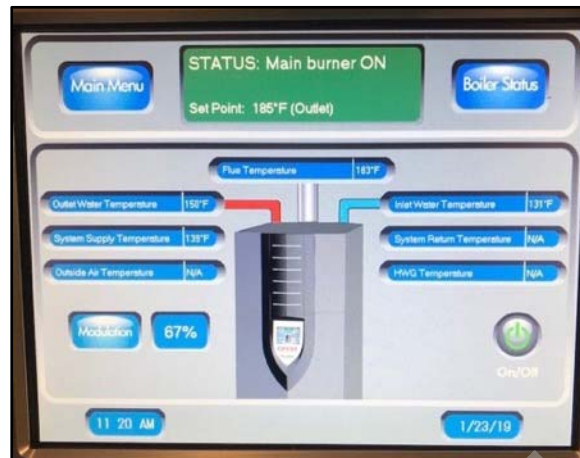
Figure 8. Control Screen for Second Boiler
