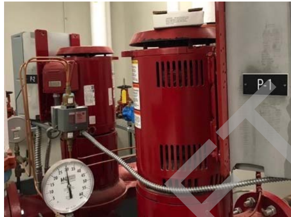
Figure 10. Heating Hot Water Pumps
