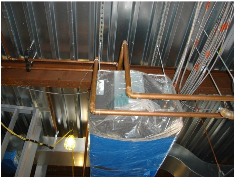
Piping in front of unit control panel
